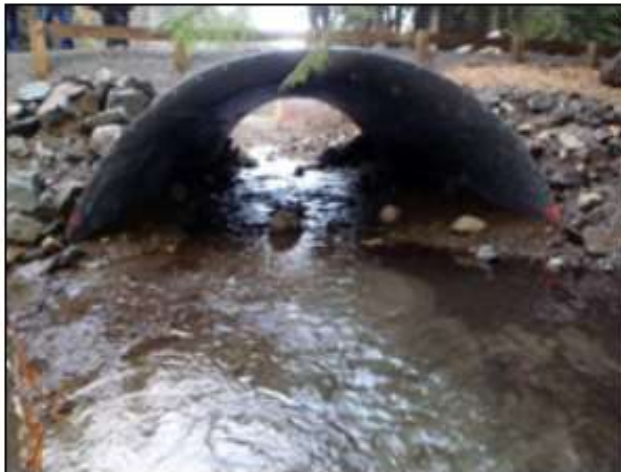
Fish can now easily swim through the new culvert on this tributary to Colville River.
