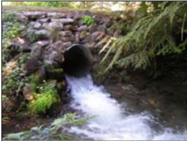
This undersized culvert increased water velocity and was a barrier to fish.
