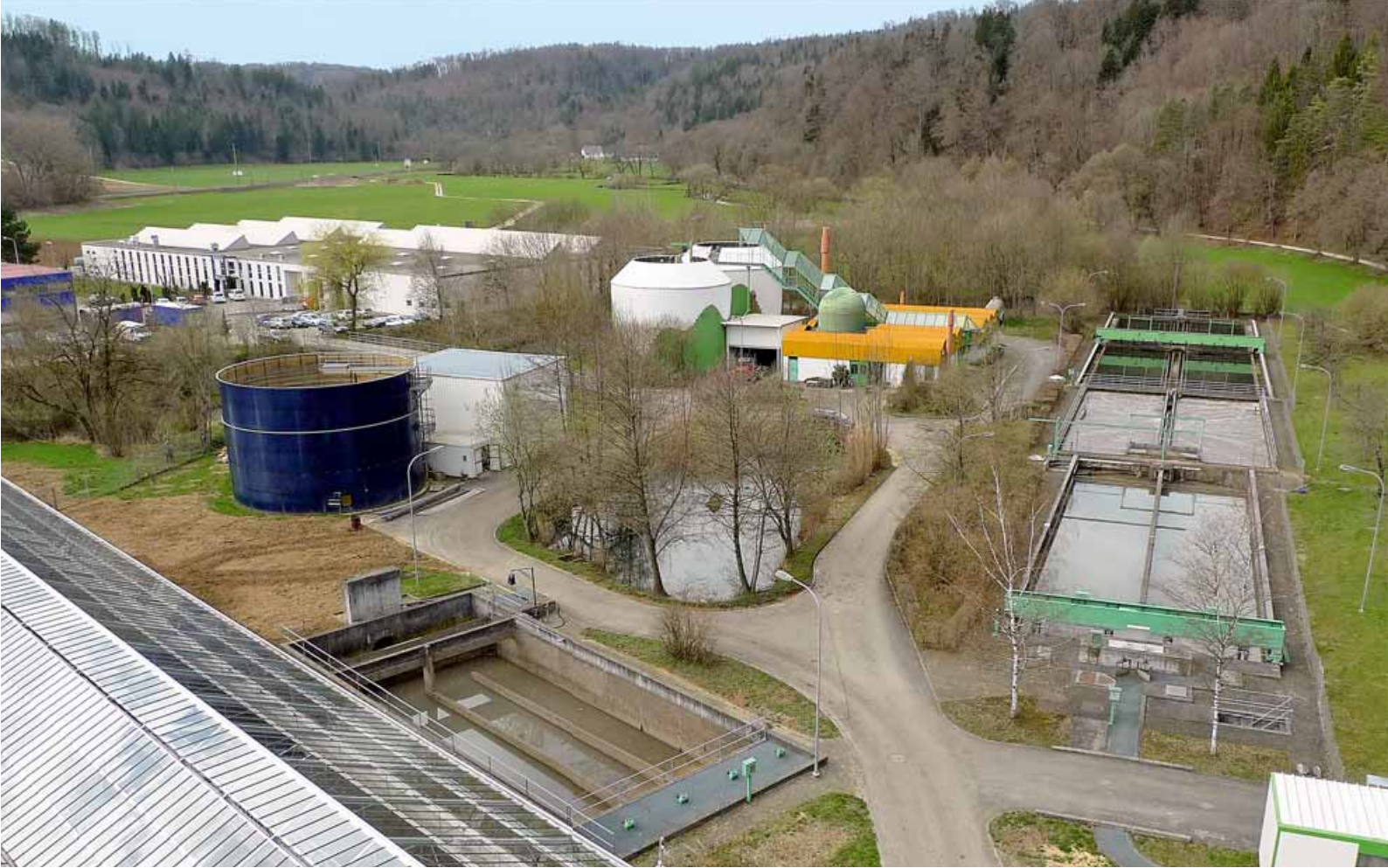
The Porrentruy wastewater treatment plant purifies the wastewater from ten communes. This cooperation increases efficiency and reduces costs.
